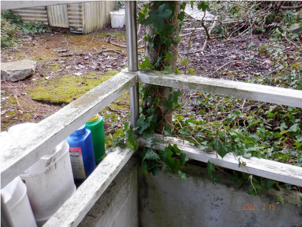
Base of Tree #890 growing up against concrete wall/steps
